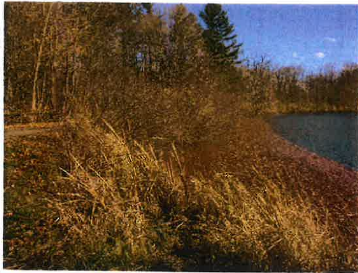
1. A view of the upstream slope from the left abutment. Note the trees, brush, tall vegetation, and cattails.
