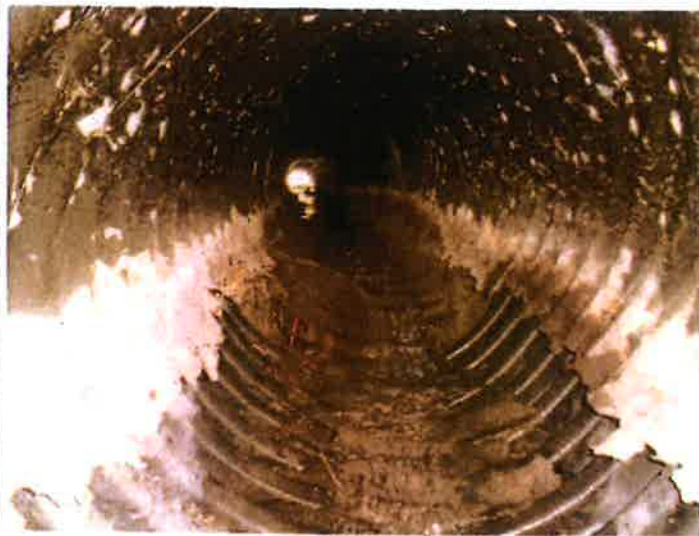
10. A view inside the aluminum CMP principal spillway outlet pipe. Note that the bottom of the pipe has completely rusted away, and the outlet is not aligned with the inlet. There also appears to be undermining for a couple feet back from the end of the corrugated plastic pipe extension.
