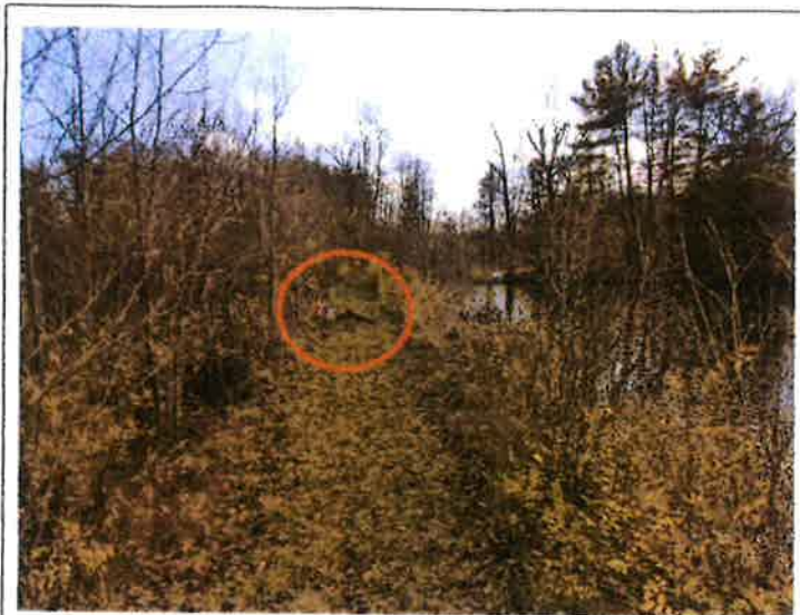
13. A view of the lake drain siphon valve located midway on the crest (circled in red).
