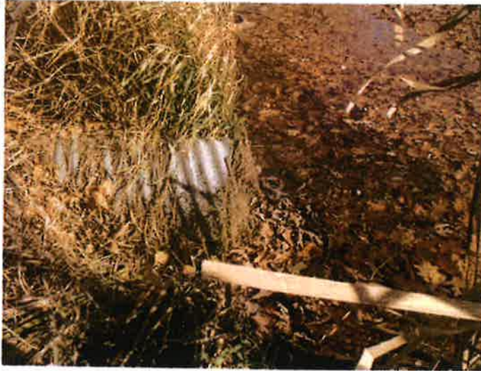
8. Principal spillway inlet pipe. Note the tall vegetation surrounding the inlet. The trash rack appears to be chicken wire staked on either side of the inlet pipe.
