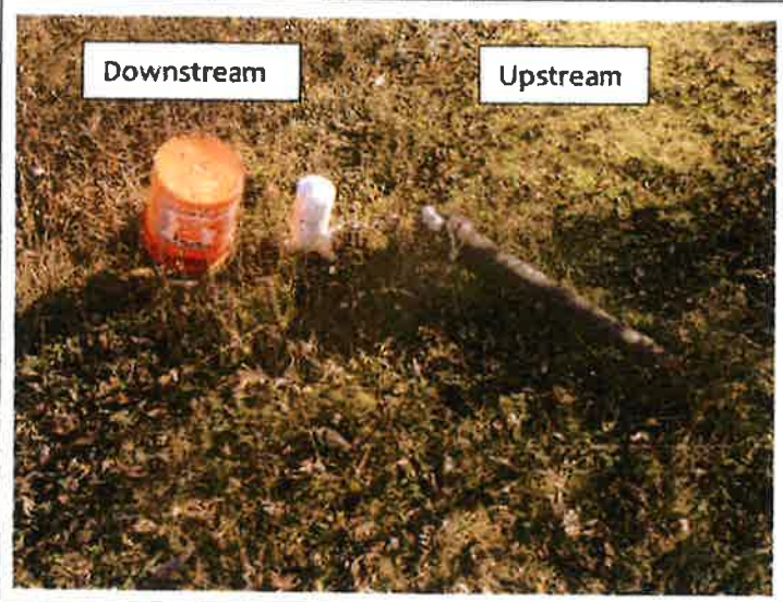
14. A close-up view of the lake drain siphon valve. Note that the siphon system consists of ductile iron pipe on the upstream side of the crest and PVC downstream of the crest. The connection is made by a Fernco flexible coupling.
