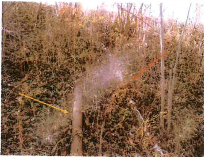
7. Another view of the downstream slope. Note the tall trees, new lake drain outlet pipe (red), and old lake drain outlet pipe (orange).
