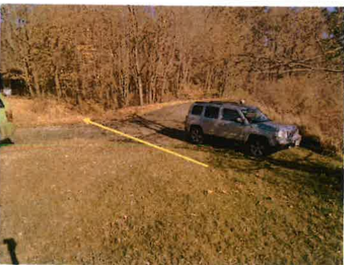
12. A view of the emergency spillway inlet, looking downstream. The yellow arrow indicates flow direction.
