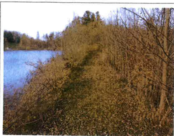
4. A view of the upstream slope from the right abutment. Note the trees, brush, and vegetation.
