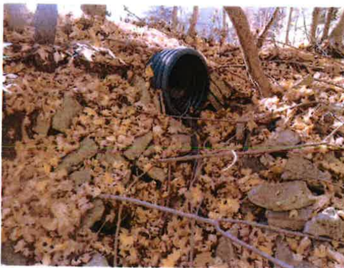
9. A view of the principal spillway outlet. Note that a short N-12 collar extension has been added to the end of the aluminum CMP.
