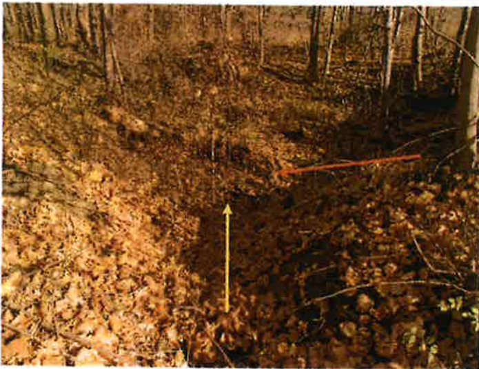
11. A view of the emergency spillway outlet channel. Flow direction indicated by the yellow arrow. The red arrow indicates approximately where the principal spillway outlet flows.
